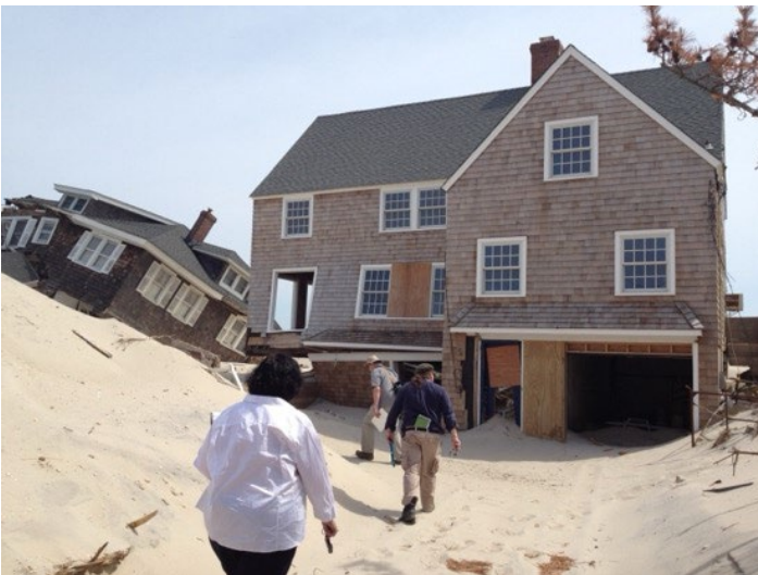
SHPO and FEMA staff survey damage after Hurricane Sandy. Courtesy of New Jersey SHPO
